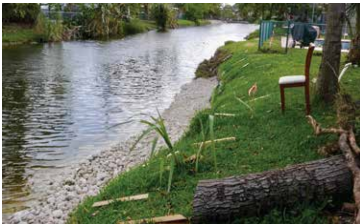
Setting up our staging area behind each home with our stakes before the material arrives.
