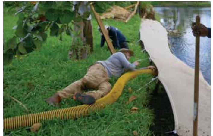
The SOX system is filled with blow-in mulch in this area behind the homes.
