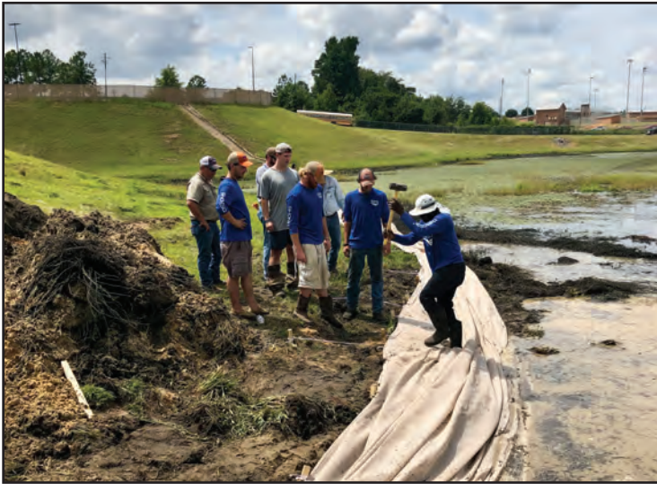
The SOX material is laid out and the staking system is pounded in place.
